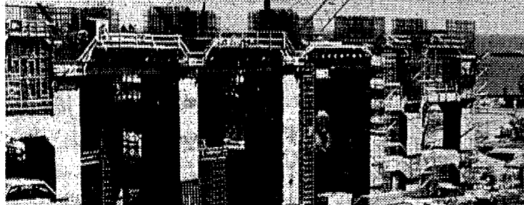
Construction at our Salem Nuclear Generating Station is well under way. Shown above is the turbine generator foundation for the first of two generator units.
