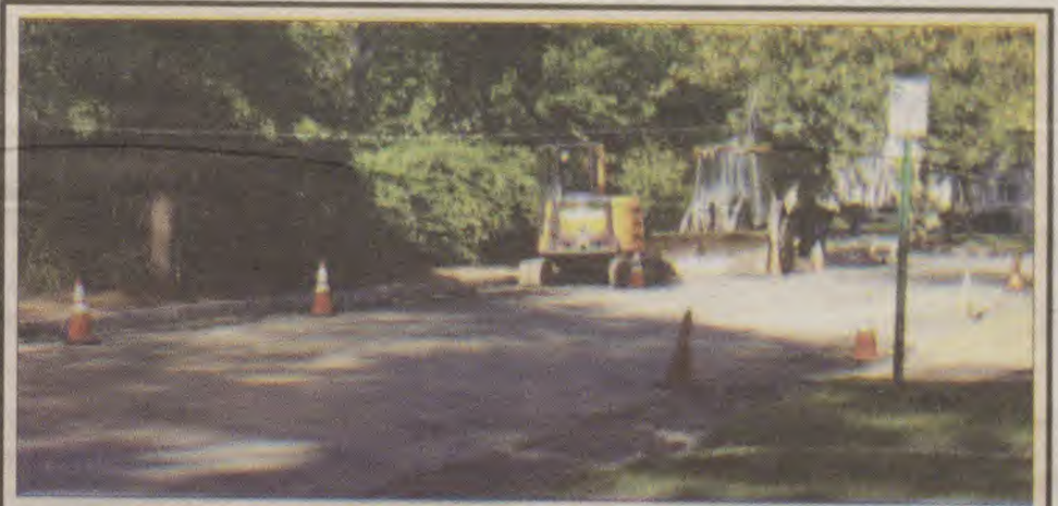
INFRASTRUCTURE IMPROVEMENTS — The Union County Freeholder's Infrastructure Grant program is under way in Fanwood, where funds will be used for roadway improvements on MacLennan Place. This year's program emphasizes road paving and improvement.
