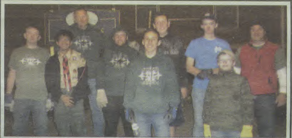
EAGLE SCOUT PROJECT — Andrew Cherego, of Boy Scout Troop 83 in Kenilworth, completes his Eagle Scout Project, building a retaining wall in front of the Kenilworth Public Library with the help of his troop Sunday, Nov. 13. Cherego raised the funds and completed the project to stop the soil erosion. From left are: Andrew Gasper, David Villafranca, troop leader John Gasper, Robbie Herbert, Cherego, Joseph Gasper, Aidan Musser, Vincent Grimaldi, and assistant Scoutmaster Rick Cherego.
